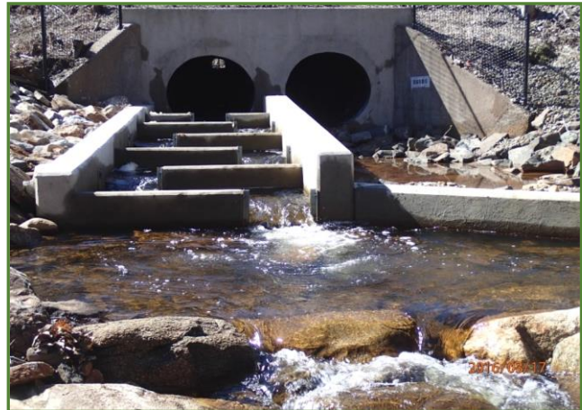
View of pool/weir fishway constructed at the tributary to Lyman Brook outlet.
